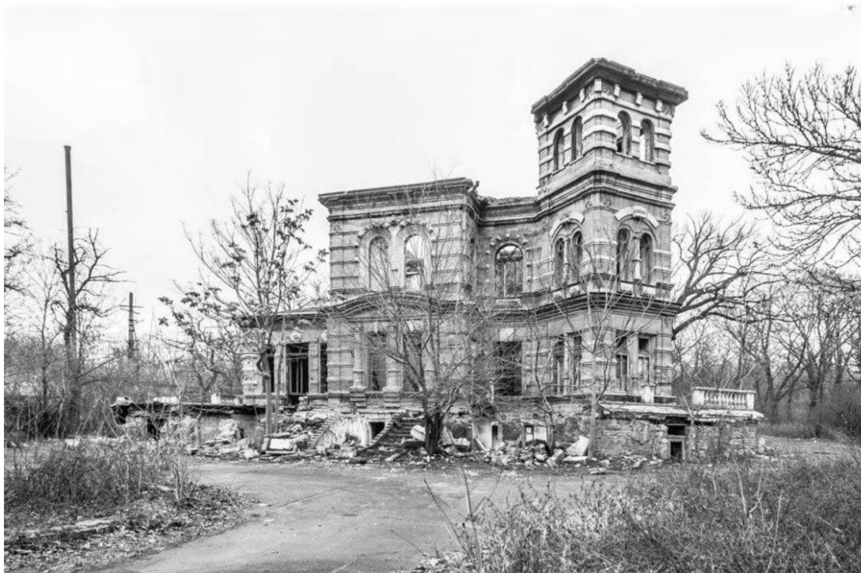
Fig. 1 An example of a structure that requires analysis and evaluation of resources, value, quantity, attractiveness, accessibility and other factors
