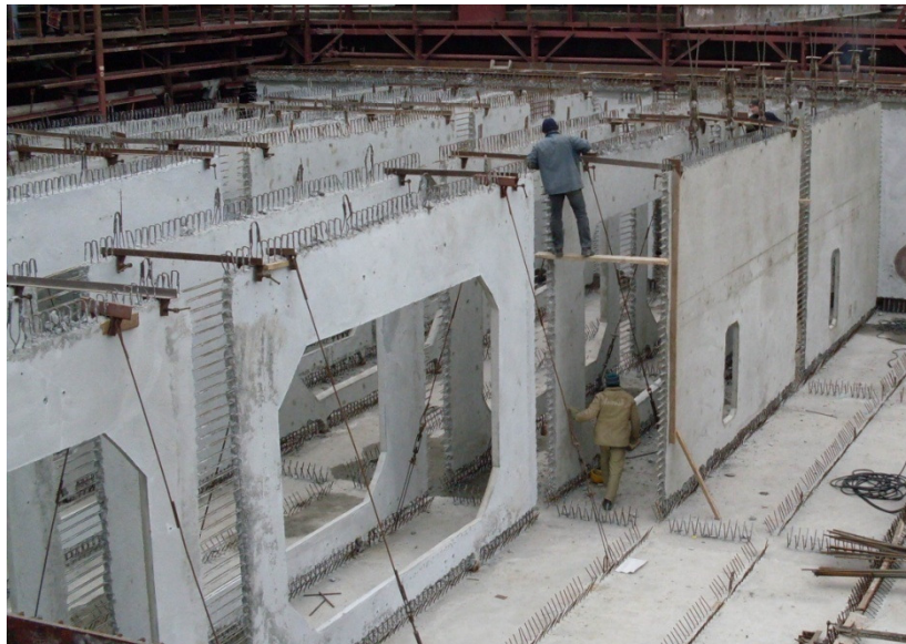
Figure 1: Construction technology of concrete floating structures at the Kherson State Plant "Palada" (Kherson, Ukraine).
